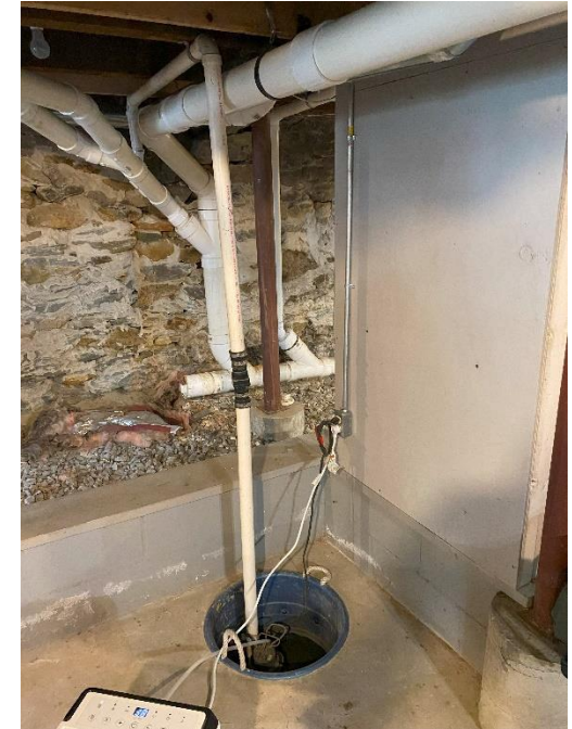
Sump Pump Discharge to Sewer
