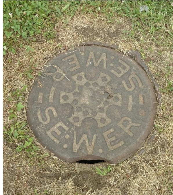
Damaged Sewer Manhole Cover
