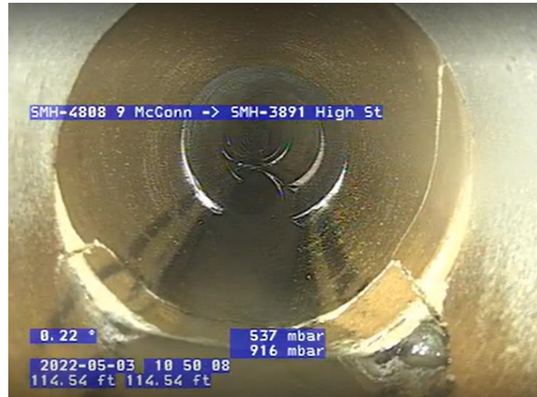
Cracks in Pipe
